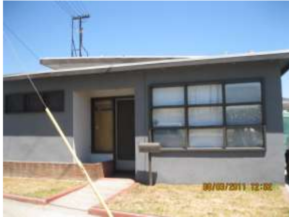
Before: Façade does not note the business name.
