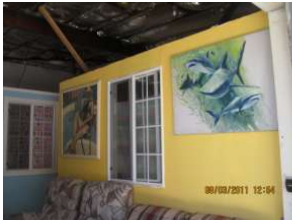
Before: Illegally subdivided living quarters.
