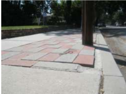
Before: Inadequately maintained parkway area.
